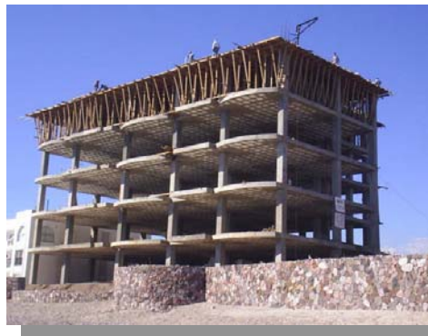
Left: Ready to pour the concrete for the roof of Building C.
