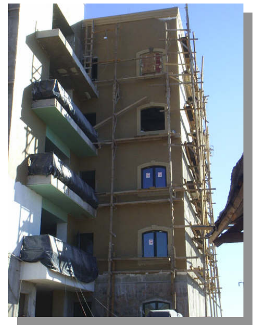
Above: West side of Building A receiving a fresh coat of paint!
